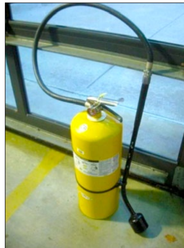
Figure 13. Class D fire extinguisher
