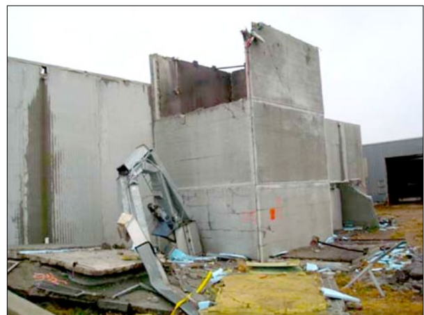
Figure 4. Coal bin explosion
