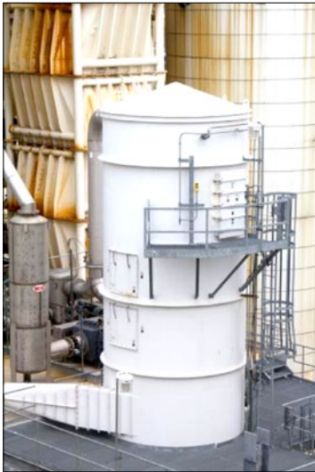
Figure 15. Access panel, walkway, and ladder on equipment
