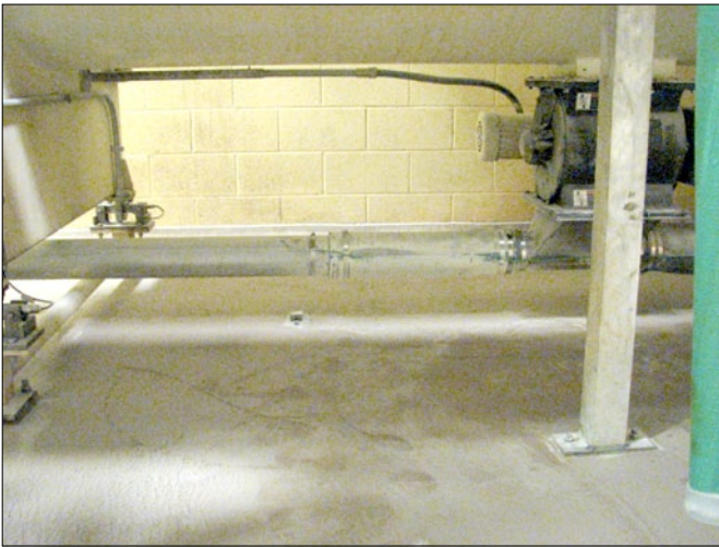
Figure 1. Conveying system piping
